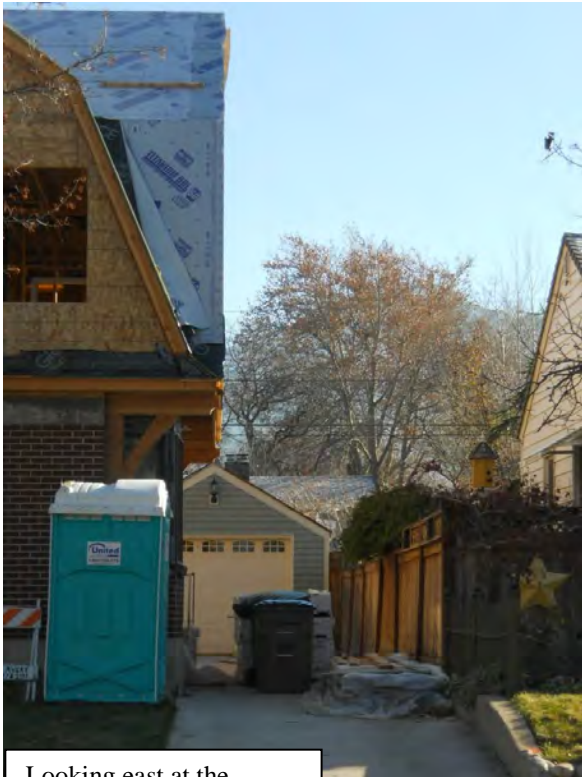
Looking east at the portion of the addition that encroaches into the side yard setback.
